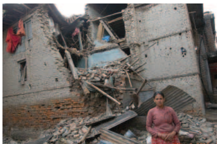
Earthquake damage in Sandku, Nepal
